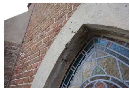
Scheuren in steen
